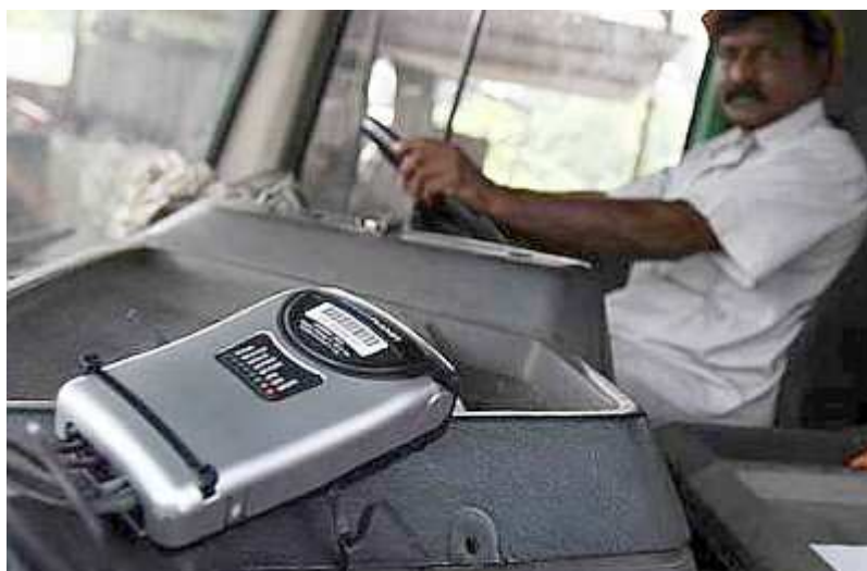
Movement tracker: An FMS device installed in the cab of a CPO tanker has saved thousands for at least one transport company.
